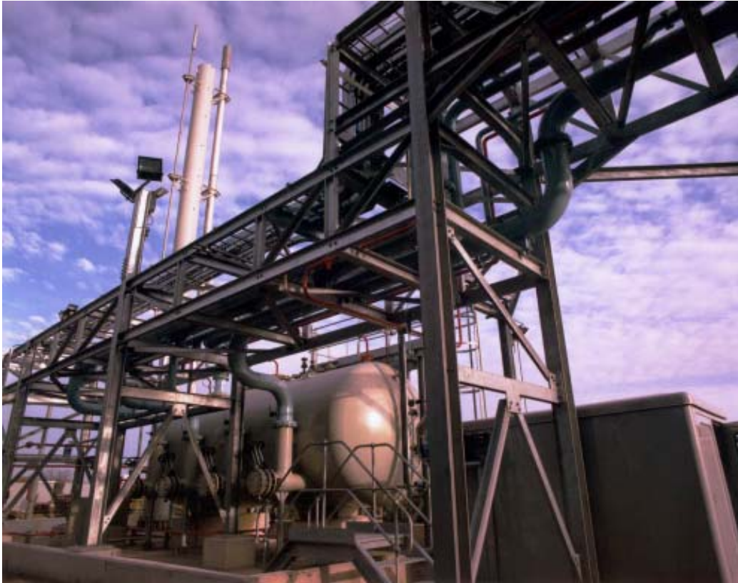
Figure 3 Quench tank installation showing inlet lines to sparges.
