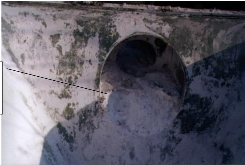
Photograph 5: Inlet to filter (from inside) showing powder accumulation
