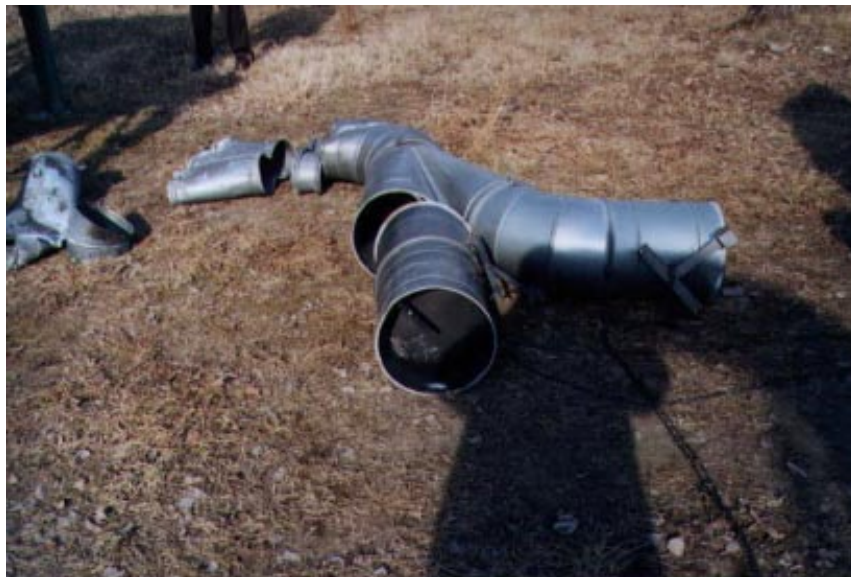
Photograph 6: Duct detail. The nearest two outlets fed the filter's two inlet ports
