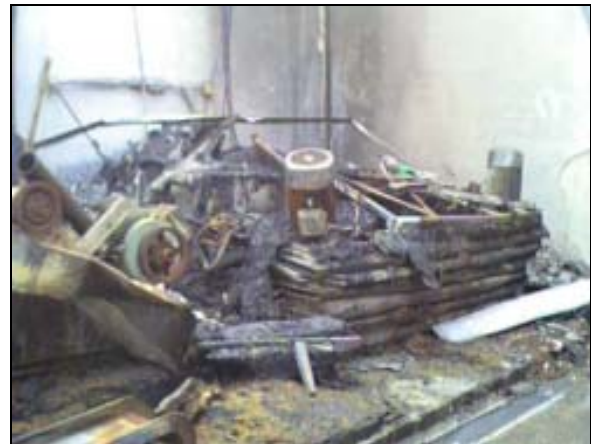
Photograph 1: Remains of a caustic water scrubber. Fires can destroy even wet systems.
