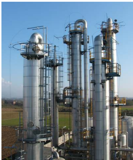
Solvent recovery plant
